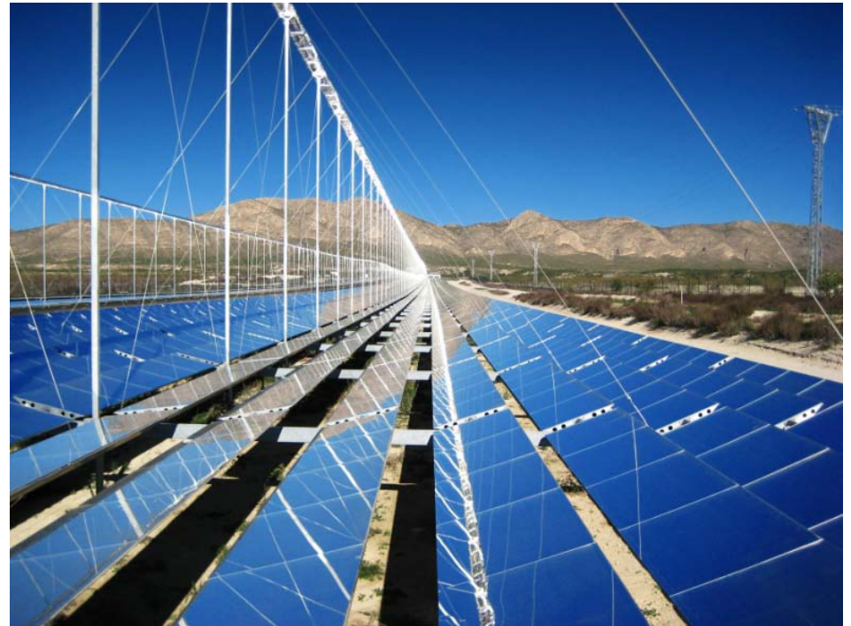
Puerto Errado 1, Turnkey Solar Boiler, Southern Spain
