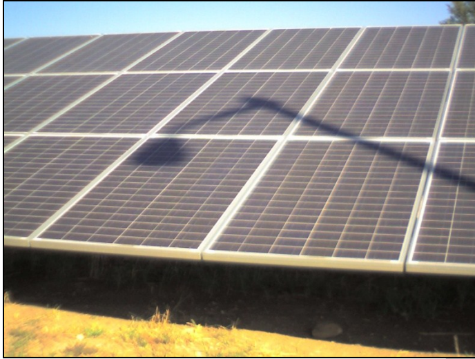
Figure 11: A nearby shading obstruction (light pole) casts a shadow across Test Array 2.
